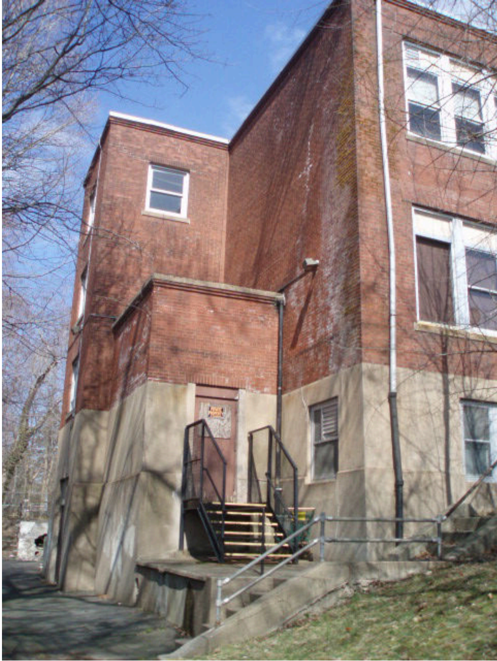
View of the south end of the school
