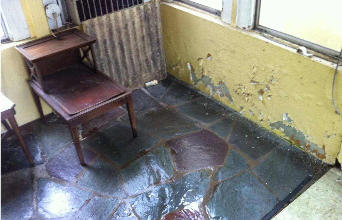
Fig. 53 – View enlarged area of breezeway. The floor is wet from active roof leaking. Note the corrugated fiberglass roof panel stored in the corner of the room which was formerly above the rear door of the breezeway. Photo taken looking east, June 2017.
