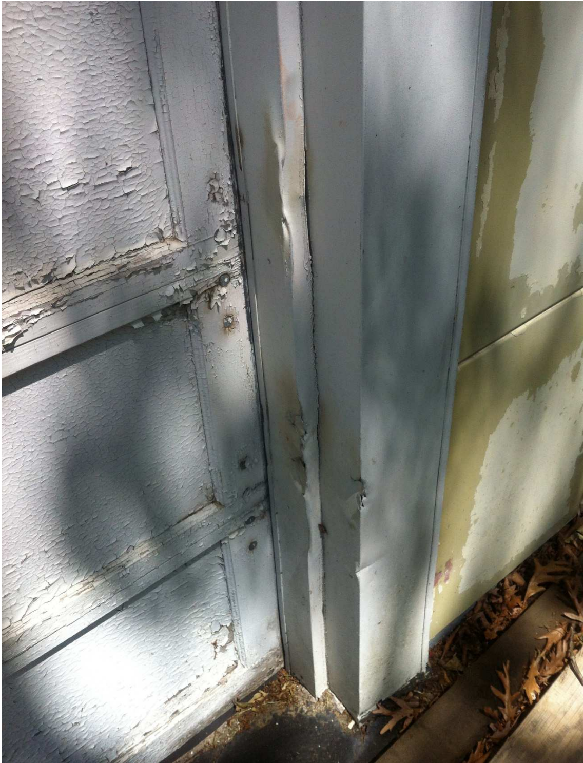
Fig. 26 –The sheet metal panning on both garage door jambs has been dented through various impacts. This material could be replaced in-kind. Photo taken looking east, June 2017.
