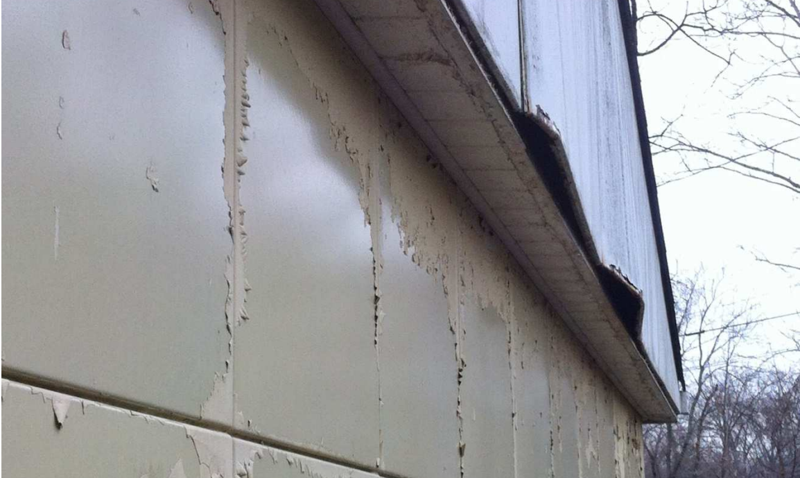
Fig. 24 – The fascia panels at the west side of the garage gable have been damaged and will need to be removed, straightened, and re-installed. Similar to the “Maize Yellow” panels, the white trim panels were also painted. The white latex paint should likewise be removed and the original finish restored, photo taken March 2017.
