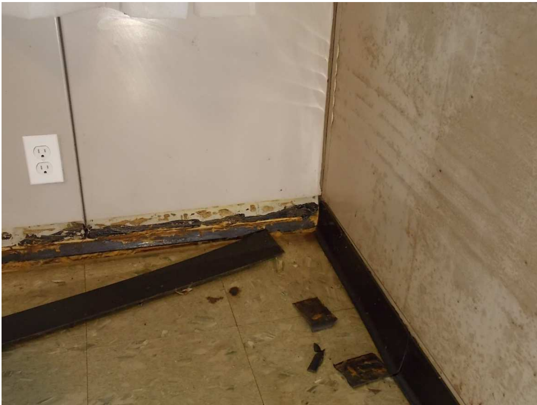
Fig. 73 – The adhesive securing the base to the wall panels has failed in many areas causing the base to fall off. These sections should be reinstalled. Missing or damaged sections should be replaced with new base that matches the original. Also note the surface rusting of the China Cabinet at right and the modern white receptacle at the exterior wall. Photo taken looking south, June 2017.
