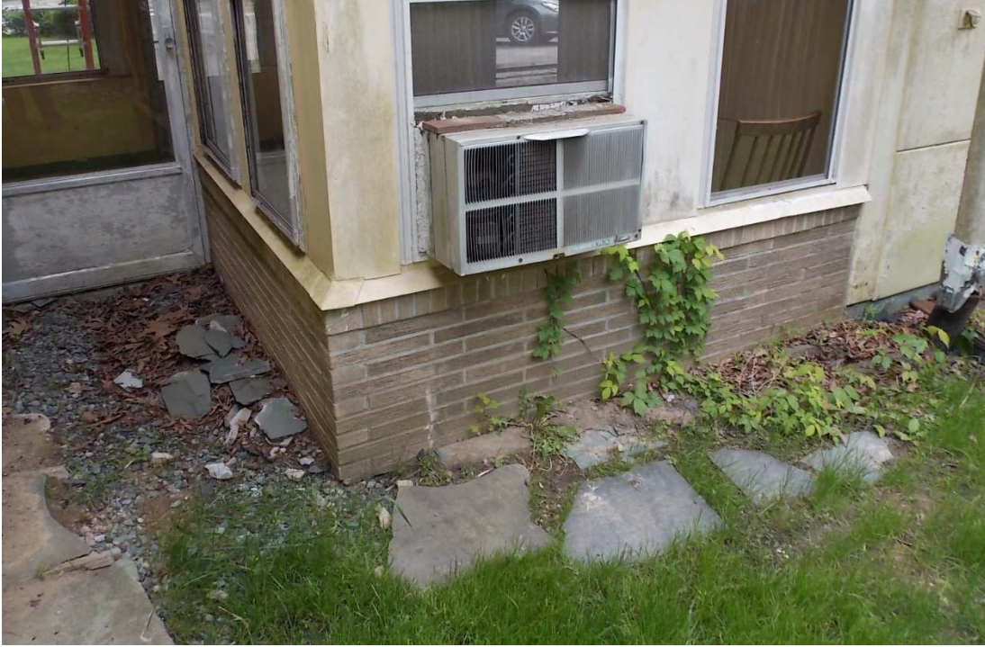
Fig. 12 – The walkway at the rear breezeway door should be restored, photo taken looking south, June 2017.
