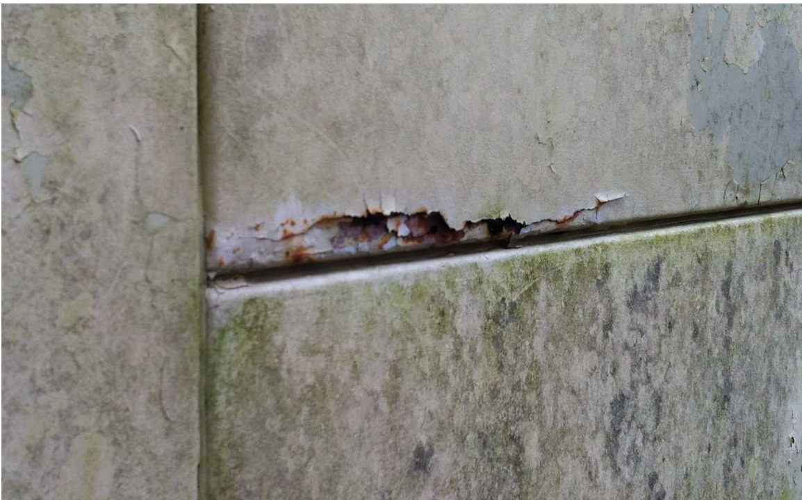
Fig. 23 – Dirt clings to the latex paint allowing algae and mildew to form. This north east corner panel has rusted through and will need to be repaired, photo taken June 2017.
