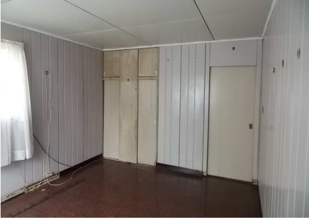
Fig. 102 – View of Bedroom No. 2, photo taken looking east, June 2017. Note the rusting of the closet and entry door.
