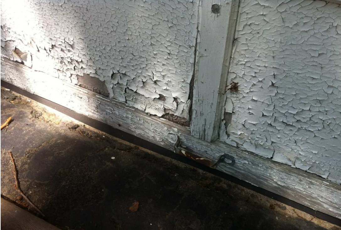
Fig. 120 – The garage door requires painting, photo taken looking north, June 2017.
