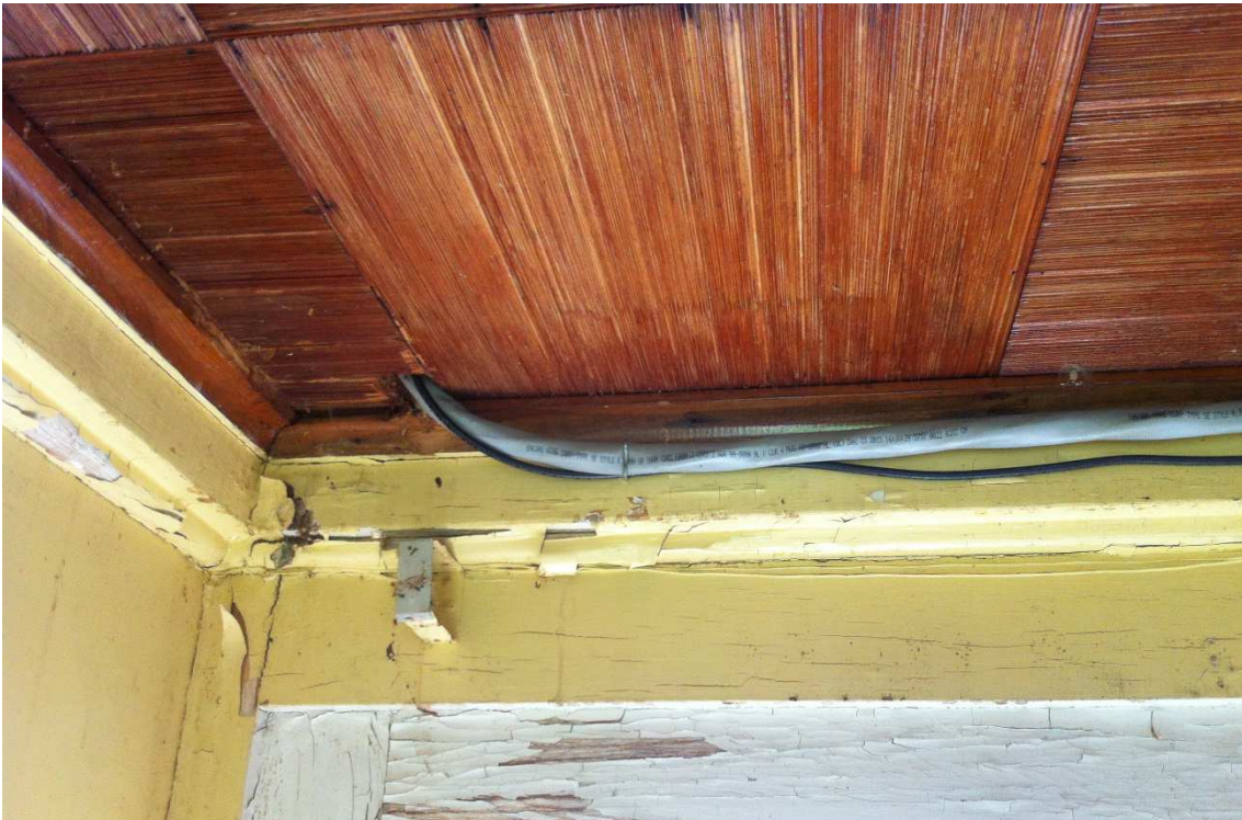
Fig. 56 – View of breezeway ceiling with new wiring, photo taken looking south, June 2017.
