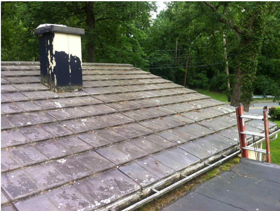
Fig. 36 – Much of the paint which was applied to the roof panels circa 1990s has worn off, there is still a rougher texture than the original porcelain enamel which catches dirt and debris allowing lichen to form. Looking south, note the paint on the chimney casing, photo taken June 2017
