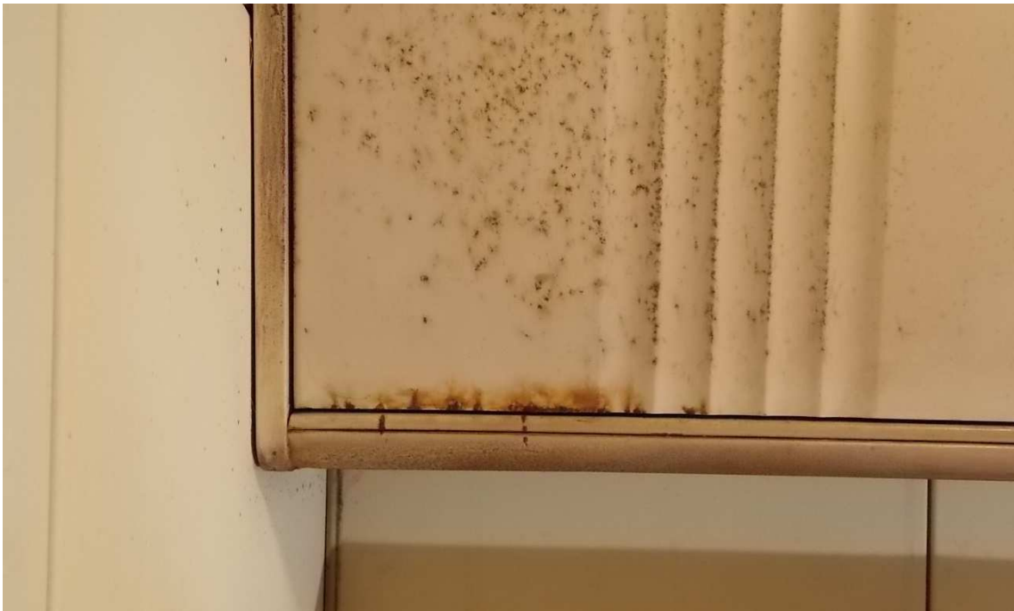
Fig. 62 – View of typical rust damage to cabinetry and closets. This is the kitchen cabinet above the stove, photo taken June 2017.
