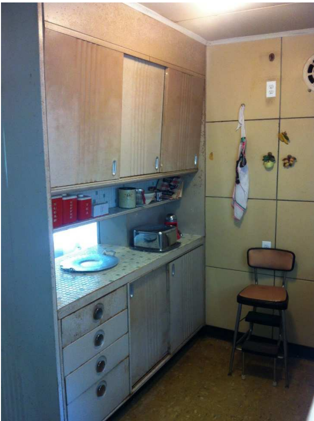
Fig. 60 – View of Kitchen / Dinette pass-through china cabinet. Note the surface rusting of cabinet finish. Photo taken looking south, June 2017
