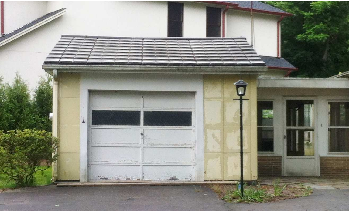
Fig. 45 – The garage roof sags at the center, photo taken June 2017 looking north.
