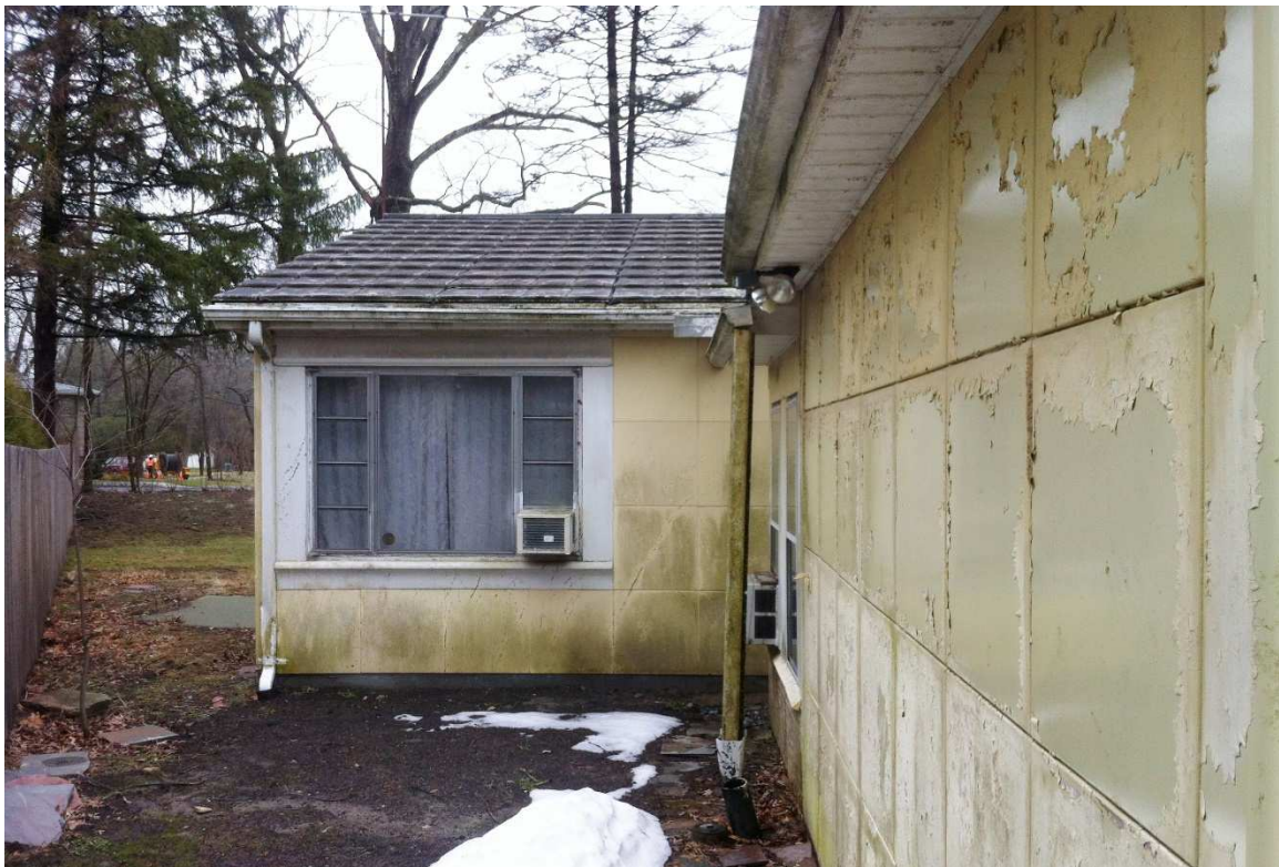
Fig. 15 – View of Bedroom 2 and rear of garage looking southeast toward Durie Avenue, photo taken March 2017.
