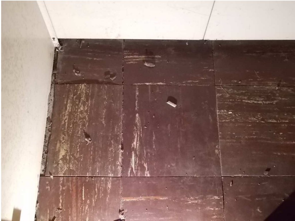
Fig. 79 – Original dark brown vinyl floor tiles located in the guest closet of the Hallway. Some need to be re-adhered. Photo taken looking south, June 2017
