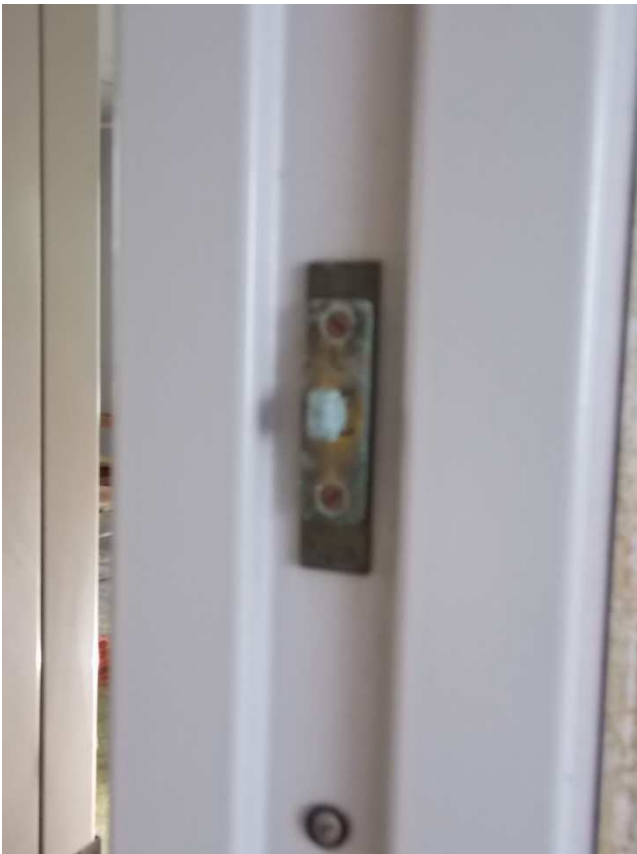
Fig. 105 – Receiver for sliding door latch, photo taken looking south, June 2017.
