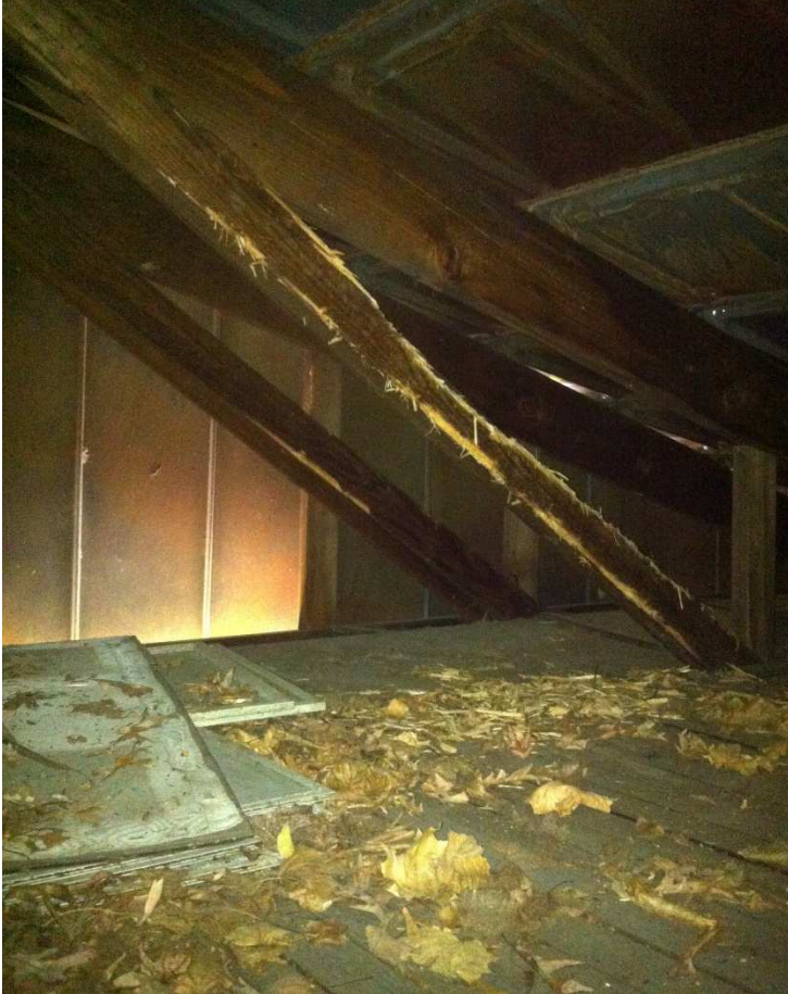
Fig. 118 – One of the truss members has been damaged by raccoon or rodent gnawing, photo taken looking west, June 2017.
