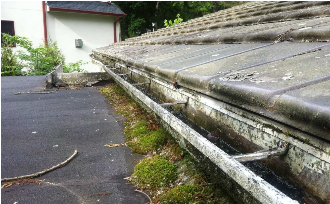
Fig. 41 – View of the breezeway roof adjacent to the house shows constant moisture has enabled moss growth. There is water damage in the breezeway ceiling below this area, photo taken June 2017 looking north.
