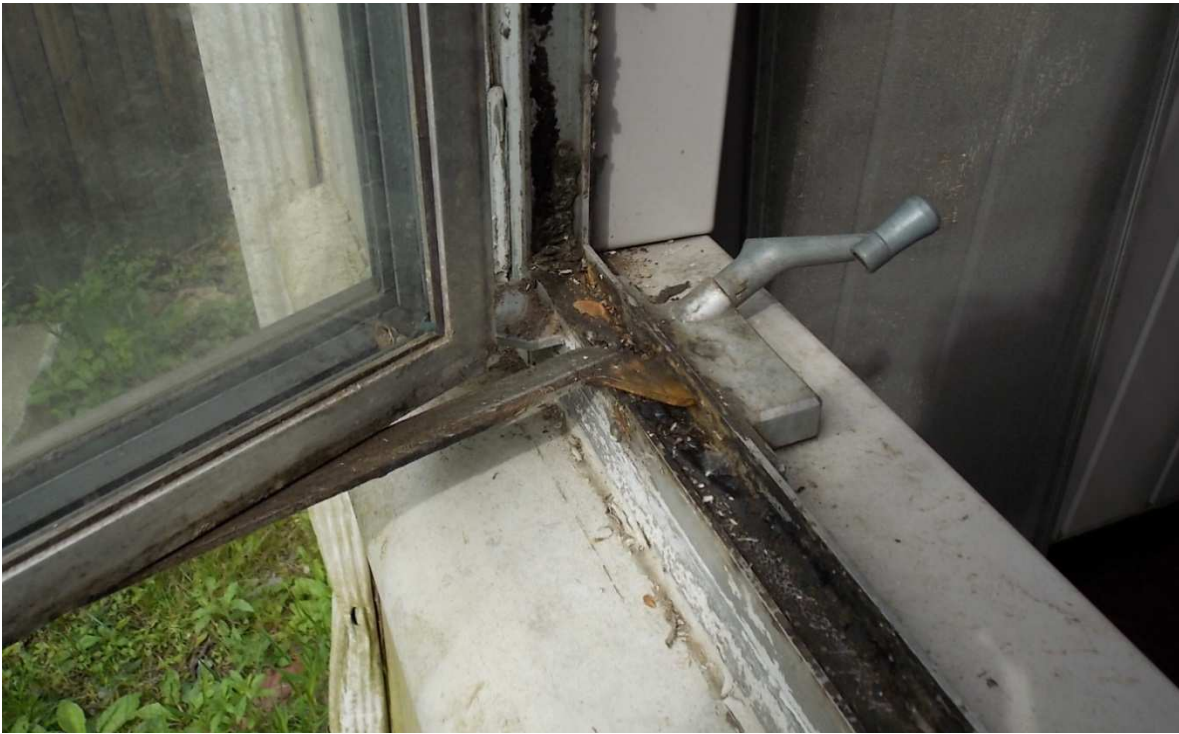
Fig. 31 – An accumulation of dirt and grime has made operation of the windows difficult on the west wall, photo taken June 2017.
