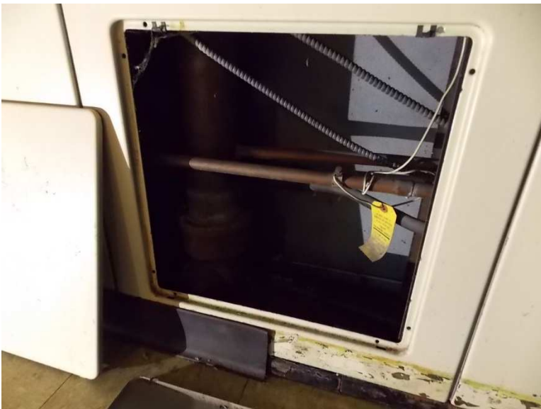
Fig. 71 – One of the access panels located in the utility wall between the Kitchen and Utility Room and the Bath. Access is provided for both plumbing connections and the electrical panel. Several sections of base are missing or damaged. Photo taken looking north, June 2017.
