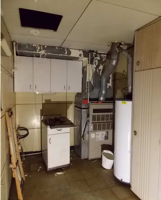
Fig. 68 – View of Utility Room looking east. Note the floor mounted furnace, exposed ductwork, non-original laundry cabinets and missing scuttle at ceiling. Photo taken June 2017
