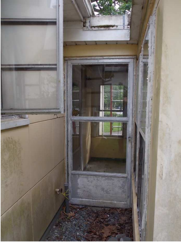
Fig. 34 –The rear breezeway door no longer opens completely due to the location of a new utility pipe. The pipe should be relocated. Photo taken looking south, June 2017
