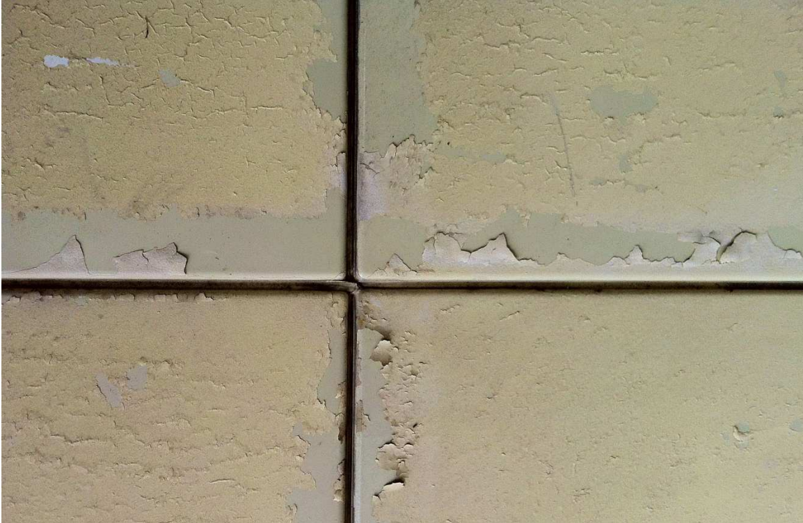
Fig. 22 – The latex paint which was applied to the exterior wall panels is peeling and should be removed, photo taken June 2017.
