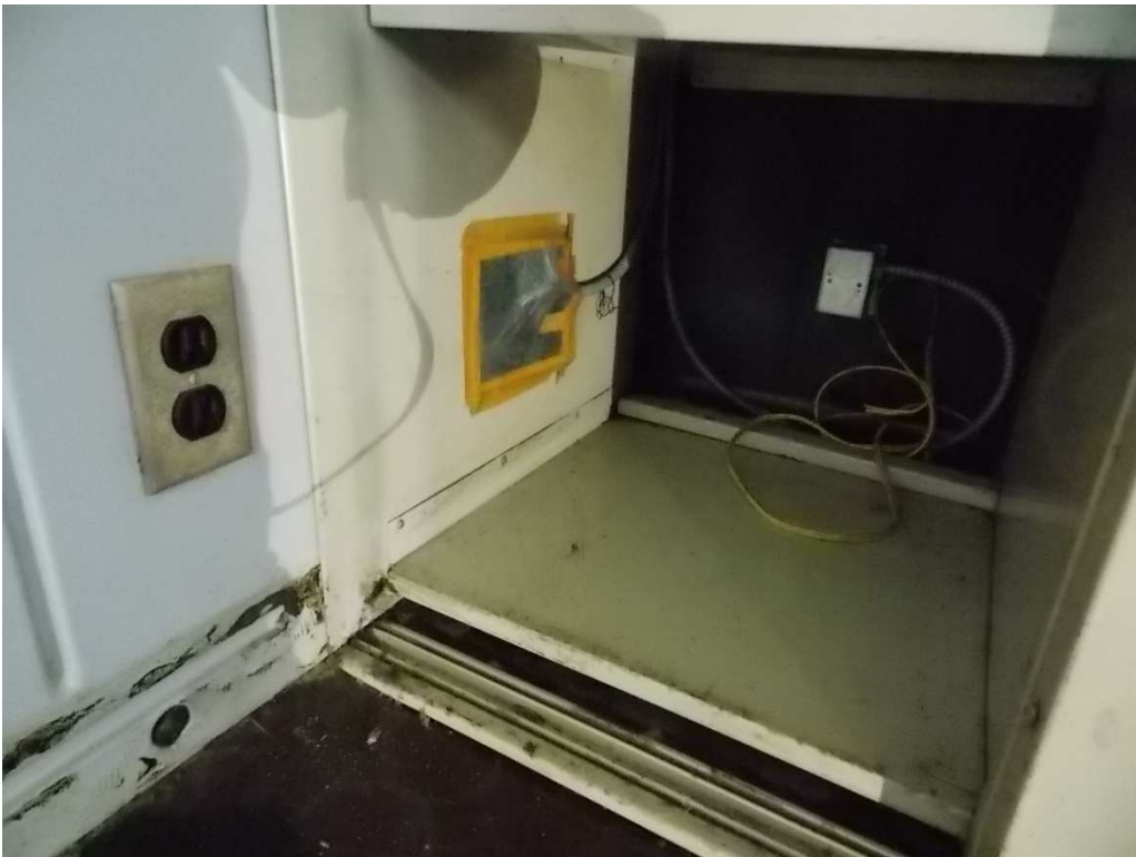
Fig. 100 – Routing of electrical wiring through the closet, photo taken looking south, June 2017.
