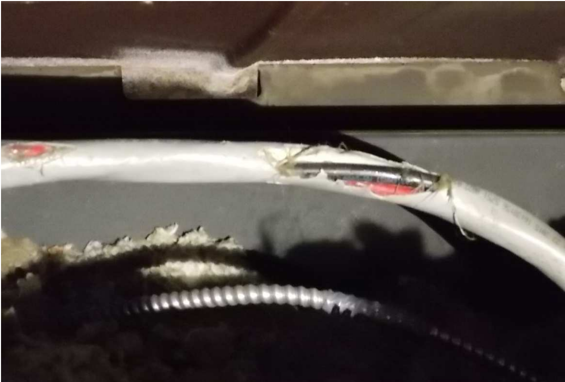
Fig. 111 – Raccoon or rodent chewed wiring, photo taken June 2017.
