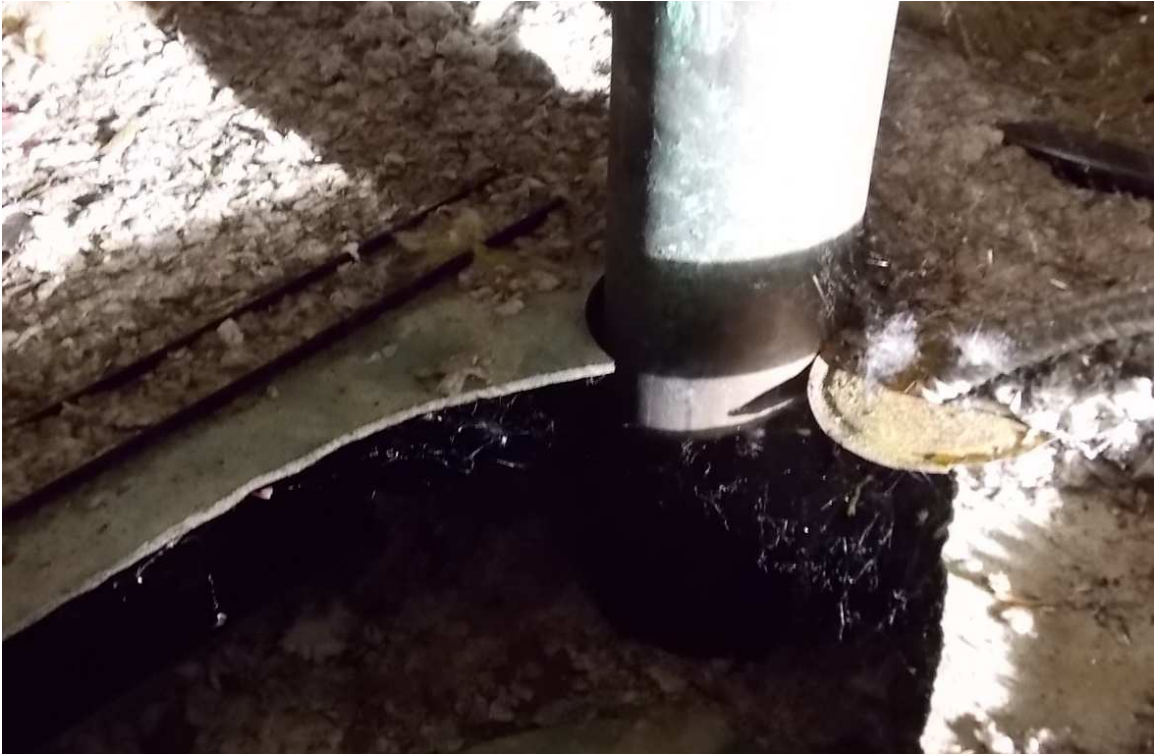
Fig. 113 – Broken cement-asbestos panel in top of plenum, photo taken June 2017.
