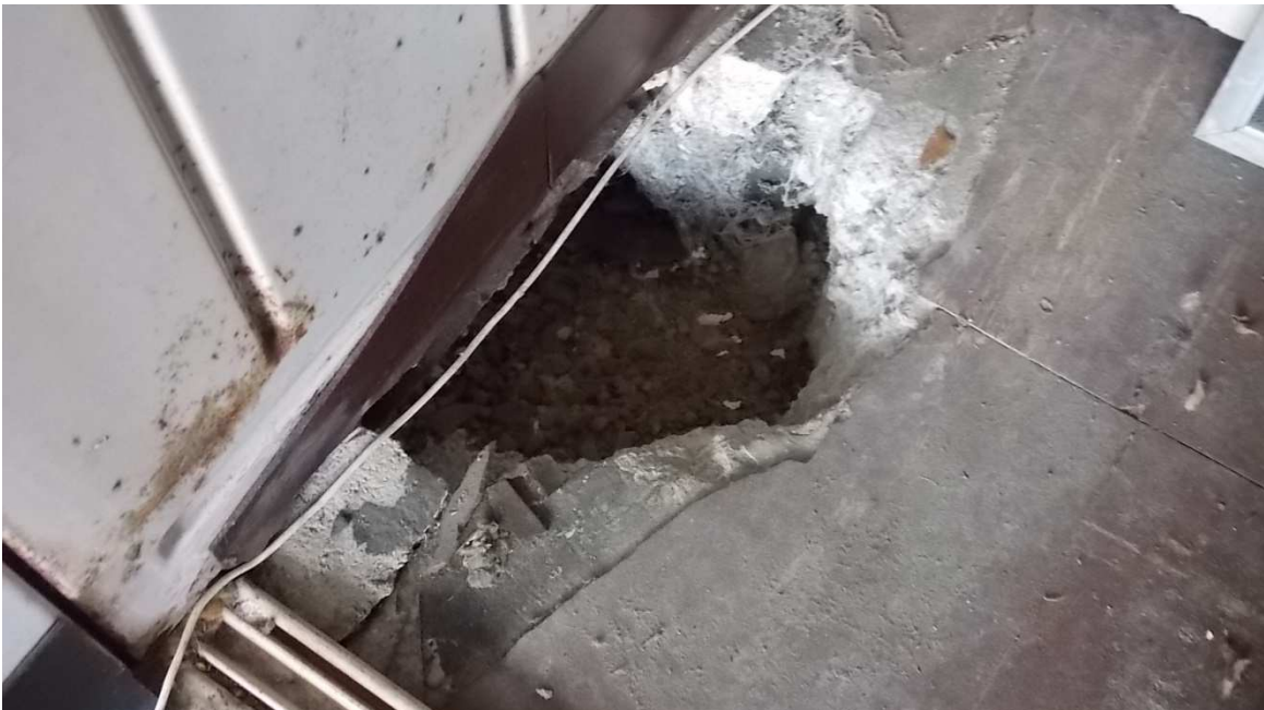
Fig. 21 – Section of concrete slab-on-grade looking north, which was removed in the Bedroom 2 closet, photo taken June 2017.
