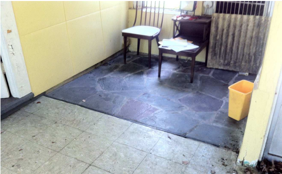
Fig. 123 – The concrete floor slab in the breezeway expansion has settled toward the rear wall, photo taken looking north, June 2017.
