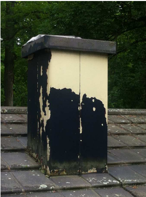
Fig. 40 – The chimney casing should have the remaining black latex paint removed and repairs made to the rust at its base. Photo taken June 2017 looking east.
