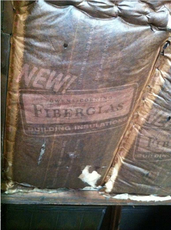
Fig. 116 – Fiberglas batt insulation which appears to date from the mid-20 th century, photo taken June 2017.
