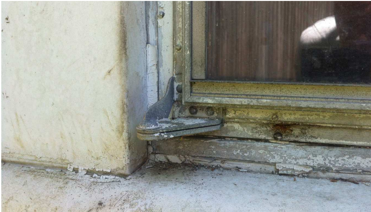
Fig. 32 –This window has had joint sealant installed at the perimeter of the steel panels. It has failed and should be removed, photo taken looking south June 2017.
