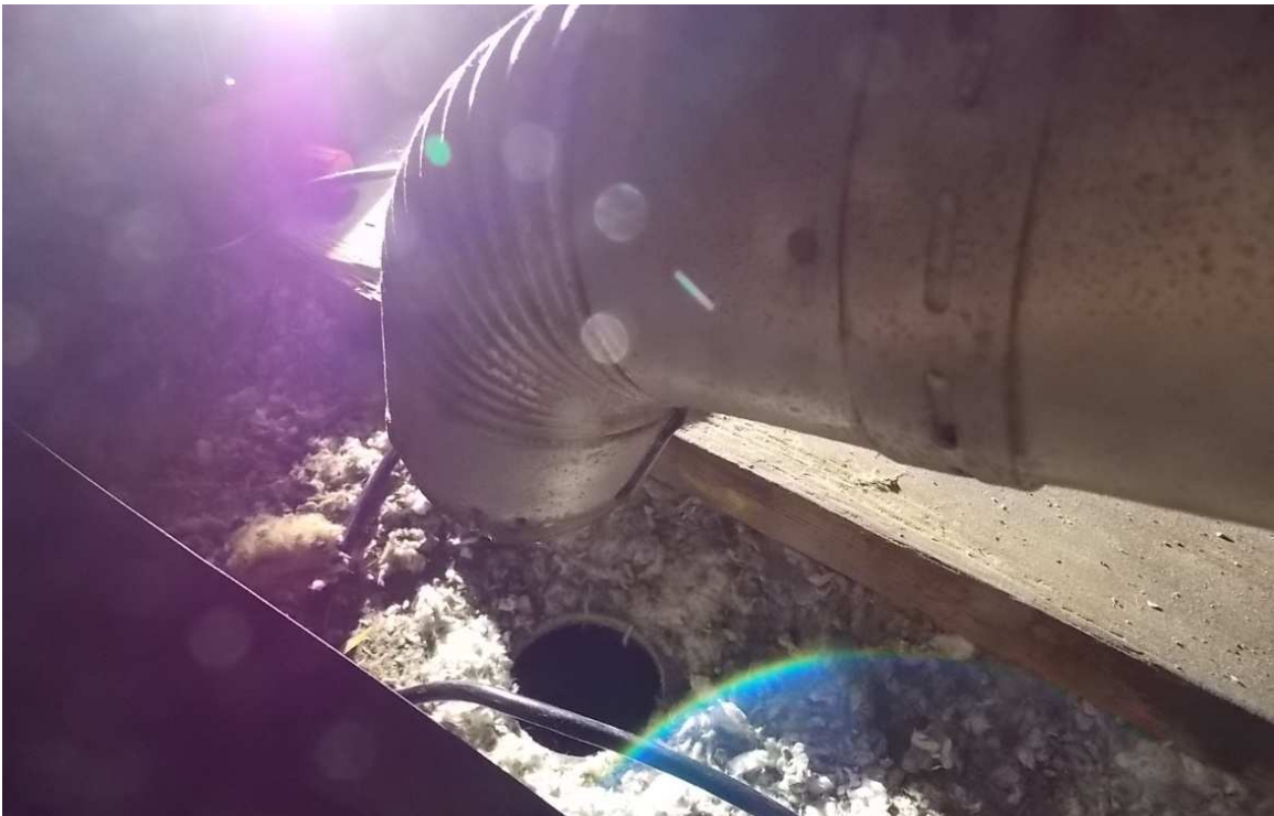
Fig. 114 – Original hole in Utility Room attic for water heater has been plugged but flue remains in attic, photo taken June 2017.
