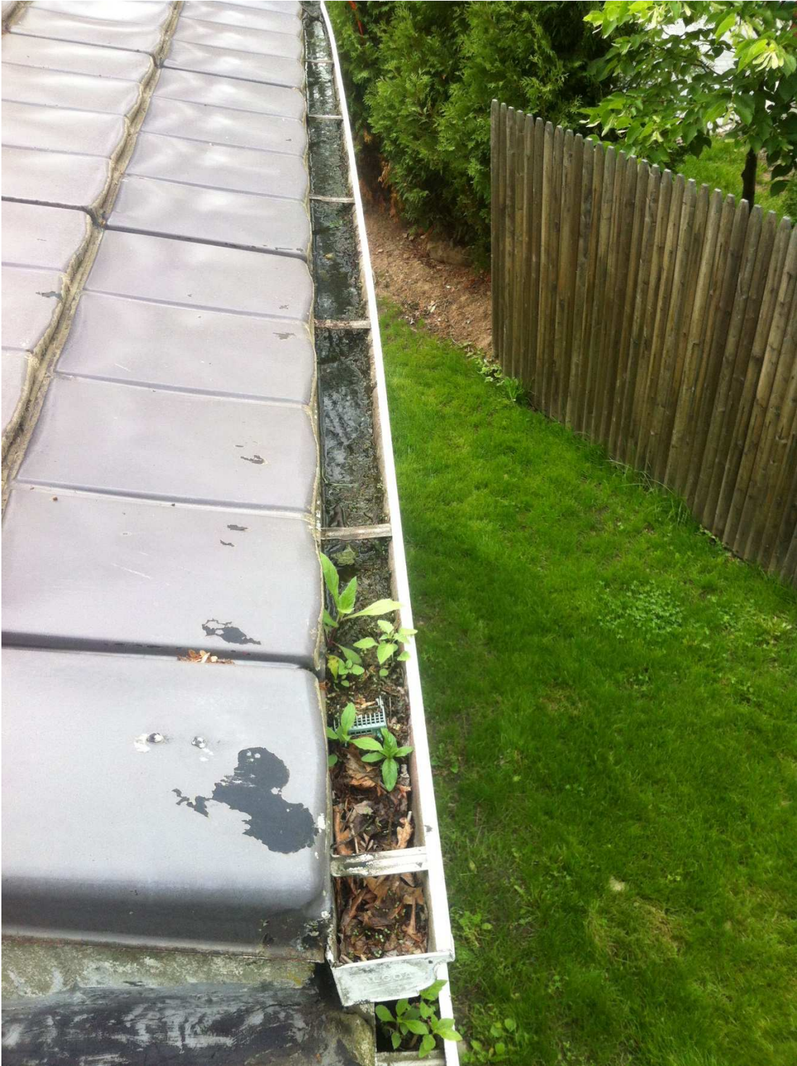
Fig. 50 – The gutters and downspouts require periodic maintenance to keep them clear, photo taken looking west, June 2017.
