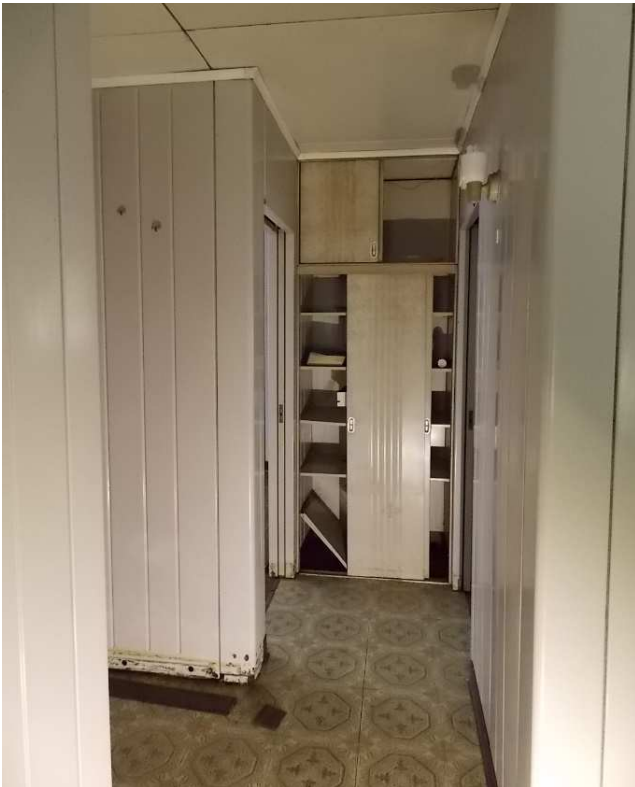
Fig. 83 – View of Hallway looking north with linen closet doors opened, photo taken June 2017.
