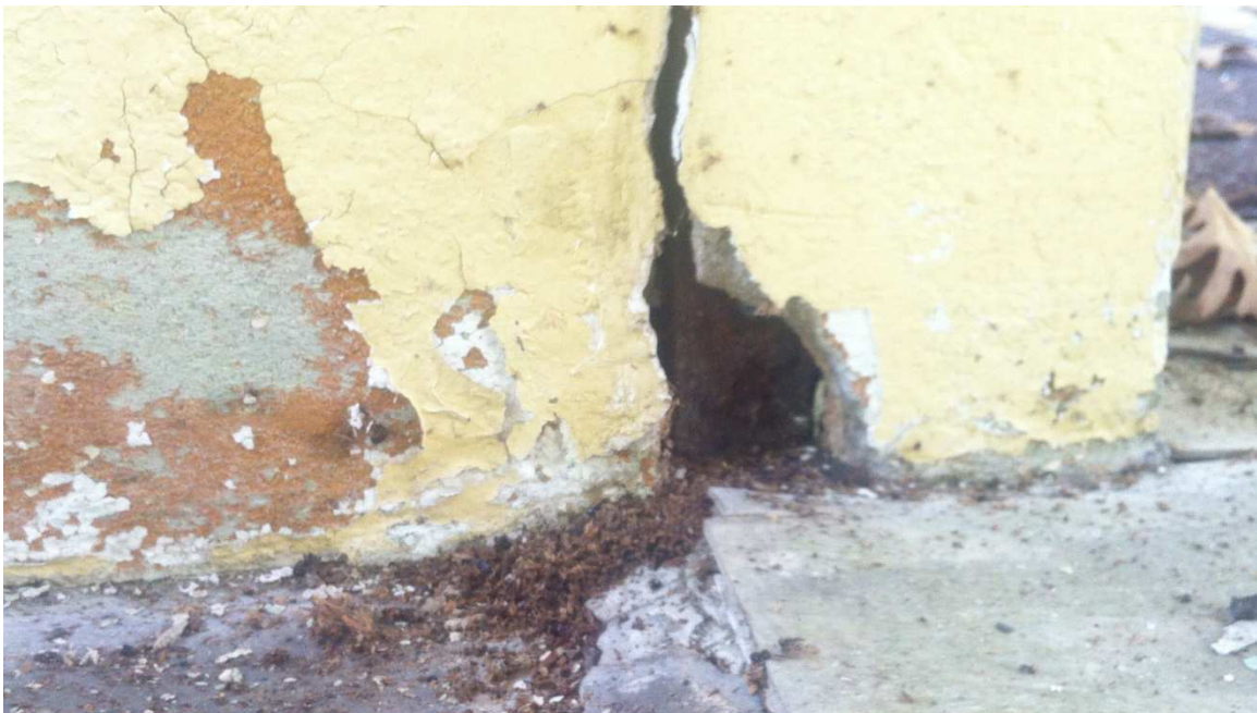
Fig. 54 – View of the base of the post adjacent to rear door of breezeway. The crack in the wall is from settlement of the rear concrete slab-on-grade. The brown material on the floor is from the base of the post inside the wall. Photo taken looking east, June 2017.
