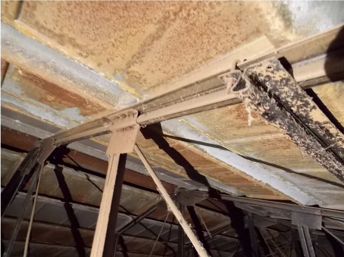
Fig. 110 – Surface rusting is exhibited on the underside of roof panels and the roof trusses.
