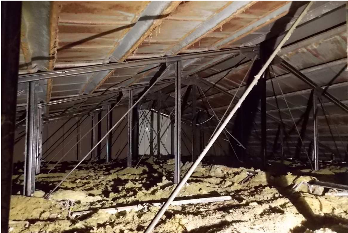
Fig. 108 – View of the attic from the scuttle location looking north, photo taken June 2017.
