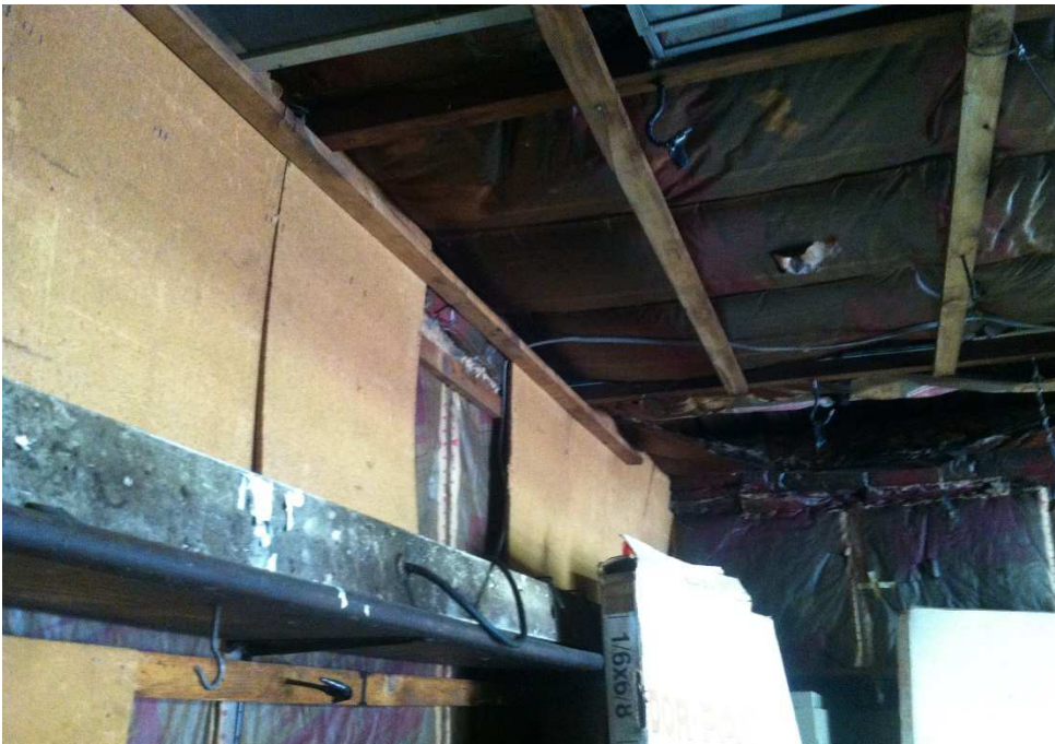
Fig. 117 – The fiberboard panels should be re-attached, photo taken looking east, June 2017.
