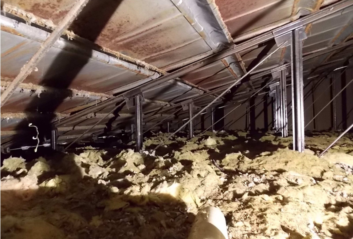
Fig. 44 – The underside of the roof panels have surface rust. The panels need to have an anti-corrosive coating reapplied to protect them from further deterioration. Photo taken June 2017 looking north.
