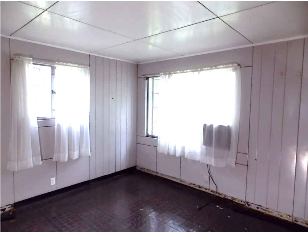
Fig. 96 – View of Bedroom No. 1, photo taken looking east, June 2017. Note the un-adhered base and shiny vinyl flooring.
