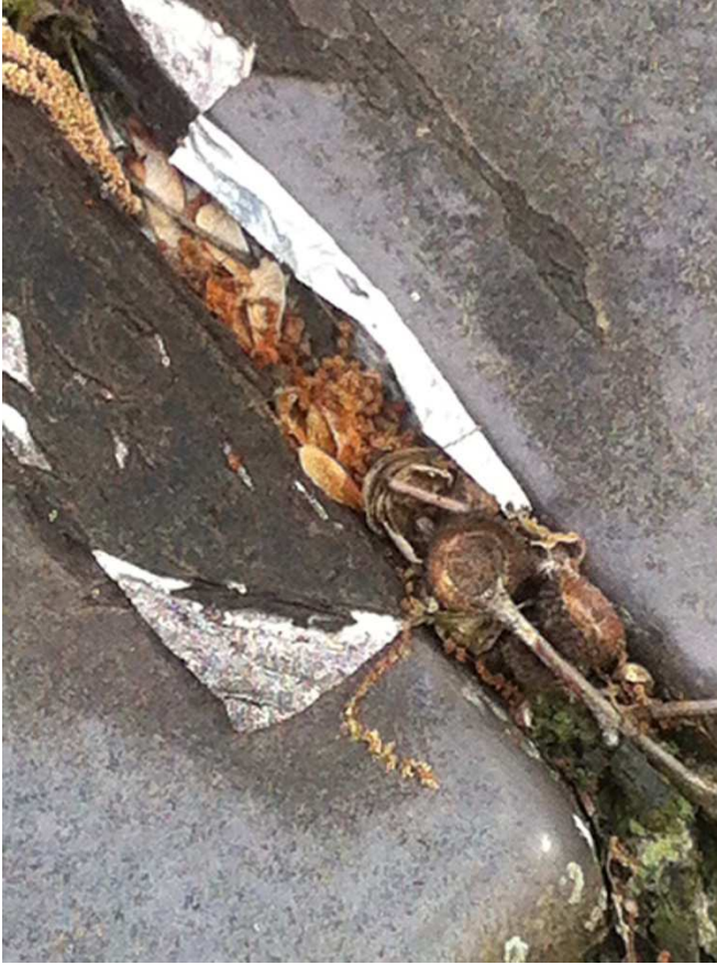
Fig. 37 – A make-shift roofing repair of metal foil and asphaltic roof coating likely covers a rust hole. The seams where the panels overlap every four feet are deeper and tend to collect leaves, twigs, and other debris which holds moisture against the panels for prolonged periods. Photo taken June 2017 looking east.
