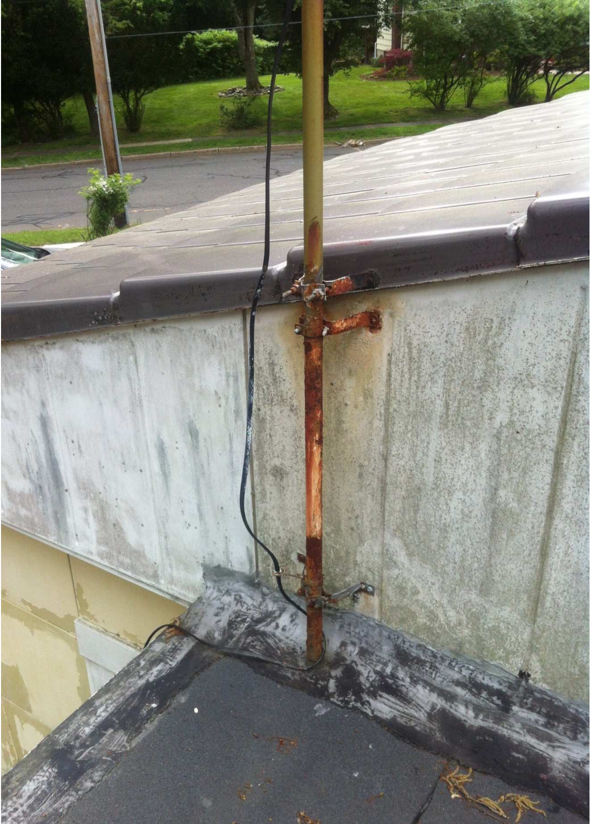
Fig. 46 – The television antennas at the garage and house are rusted. These features are important to interpret post-World War II life in America and should be retained and restored. Photo taken looking south, June 2017.
