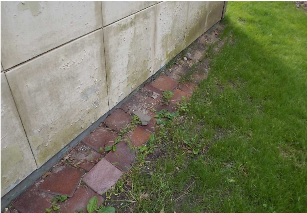
Fig. 13 – The vitreous clay tiles along the garage foundation should be reset, photo taken looking west, June 2017.
