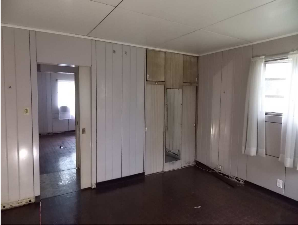
Fig. 97 – View of Bedroom No. 1 looking west toward Bedroom No. 2, photo taken June 2017. Note the deteriorated finish on the closet.
