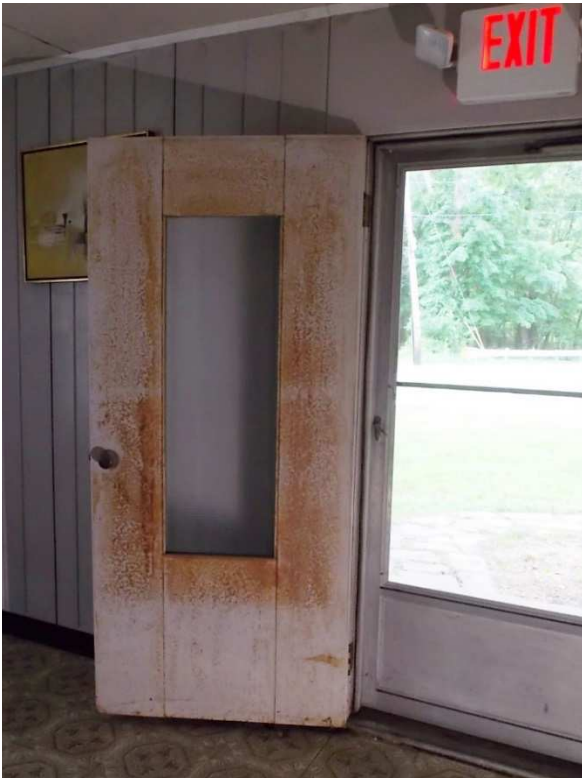
Fig. 33 –The front entry door is badly rusted and its finish should be restored.
