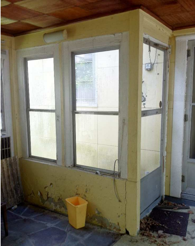
Fig. 29 –View of two of the double hung aluminum windows installed in the breezeway looking east, photo taken June 2017
