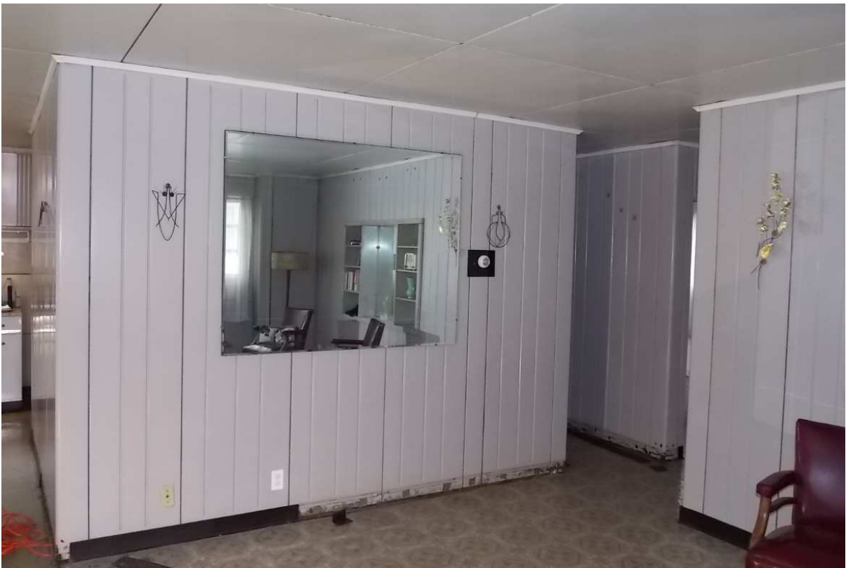
Fig. 78 – View of Living Room looking west toward the Hallway, photo taken June 2017. Note the missing section of base.
