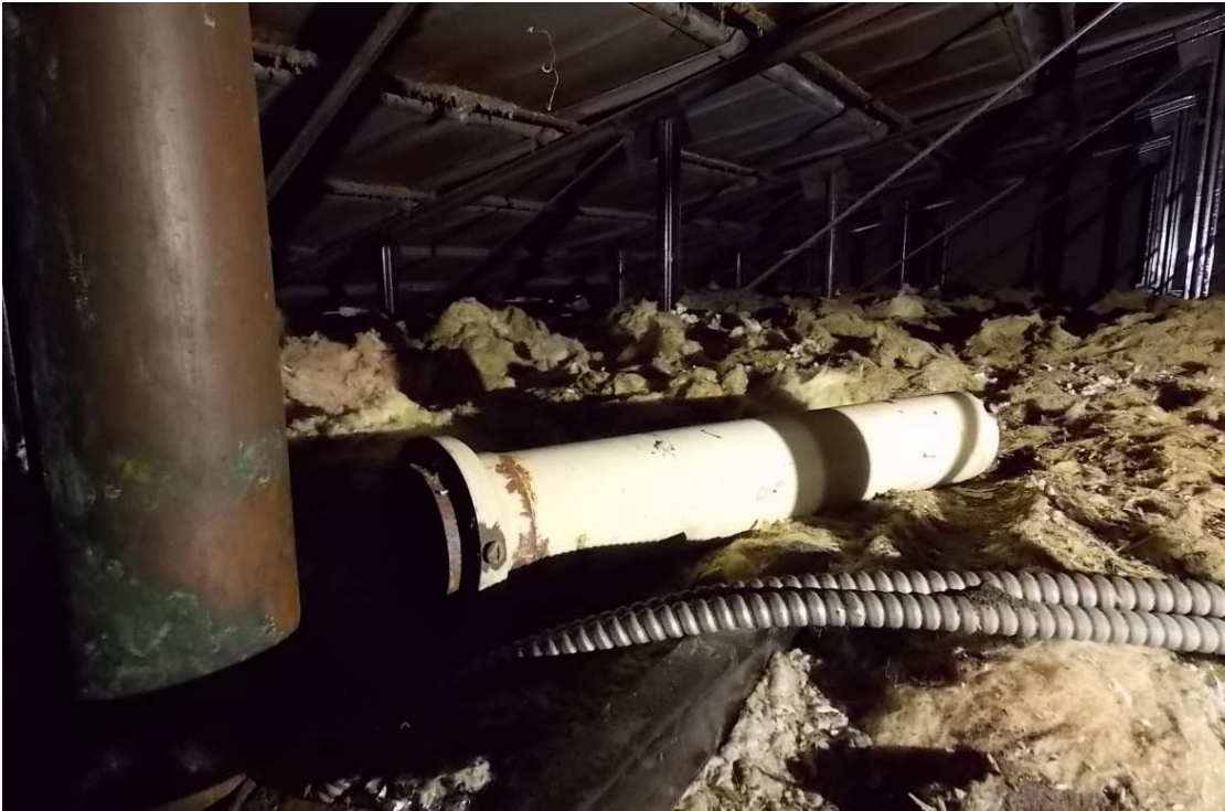
Fig. 112 – Original porcelain enamel plumbing vent remains in attic, photo taken June 2017.
