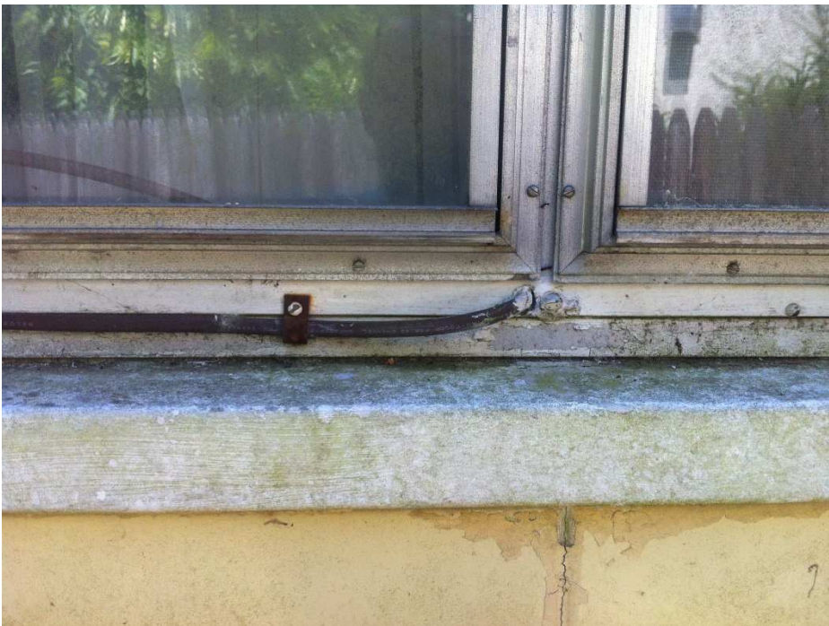
Fig. 30 –The attachment of this wire with a steel clip has caused galvanic action between the steel and the aluminum. Any attachment must isolate dissimilar metals. This should be replaced with an aluminum clip, photo taken June 2017.
