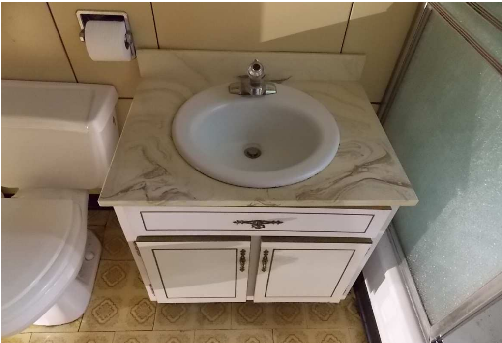
Fig. 89 – Replacement vanity sink, photo taken looking south, June 2017. See Figure 84 on page 104 for view of an original lavatory.
