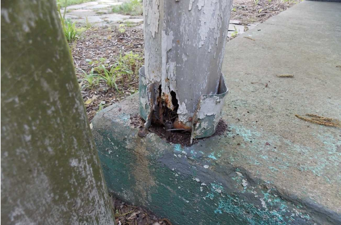
Fig. 122 – The base of the porch column is rusted and requires repair, photo taken looking west, June 2017.
