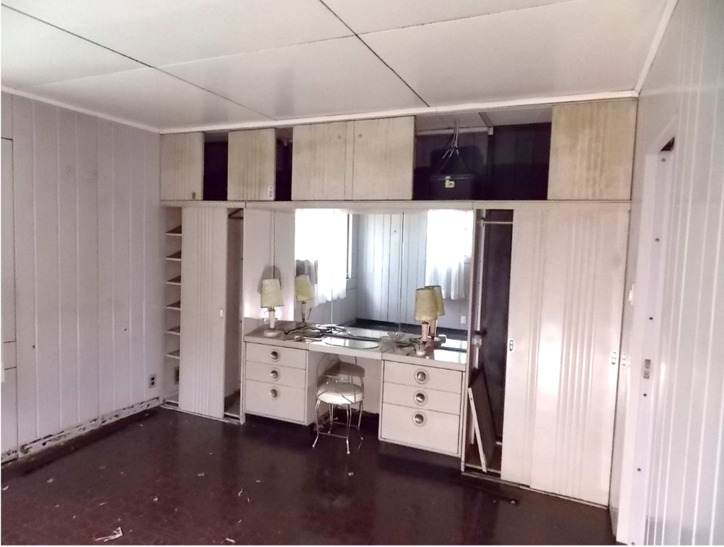
Fig. 95 – View of vanity and closets in Bedroom No. 1, photo taken looking south, June 2017. Note the missing doors.
